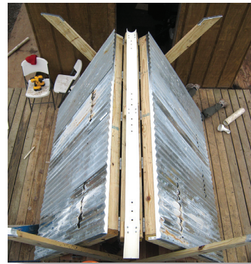
Rain collection trough to feed 'water wall'
